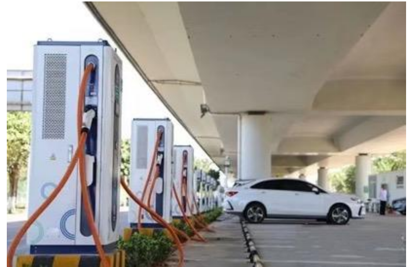
Haikou actively improves the layout of new energy vehicle charging piles.
