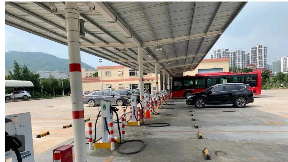
New Energy Vehicle Charging Station 新能源汽车充电站
